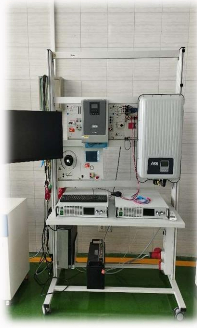
Photovoltaic Hybrid System with Battery
